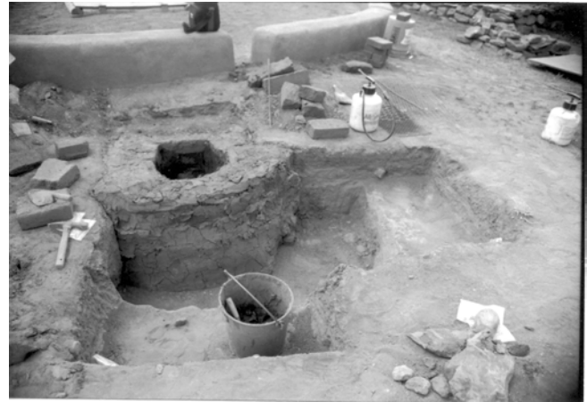
Adobe walls of Kiva 23 ventilator shaft after being repaired, Pecos National Historical Park.
