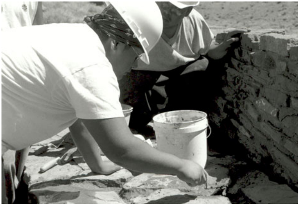
Hopi & Zuni youth repair walls at Wupatki Pueblo, Wupatki National Monument, AZ.
