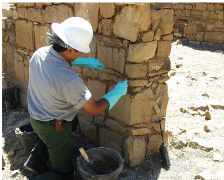
Calvin Chimoni repairs damage to the Garret Homestead, a 19 th century structure, at El Malpais National Monument, NM.
