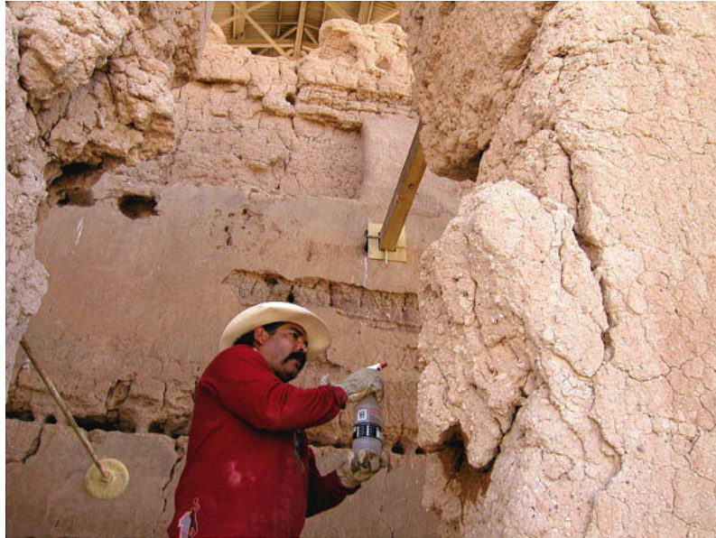
Adobe Mason Ray Madril from Tumacacori National Historical Park, AZ. repairs 700- year- old adobe walls at Casa Grande Ruins National Monument, AZ.
