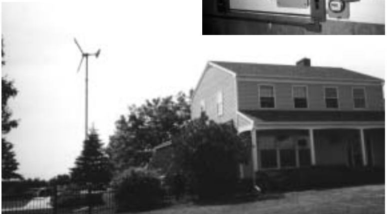
A Bergey XL.10, 10-kW wind turbine is part of a grid-connected wind/photovoltaic hybrid system that reduces the utility power used by this home in Vermont. The balance of system (upper right) includes from left to right, a Trace inverter for the PV system, a breaker box, and a Powersync inverter for the wind system.
