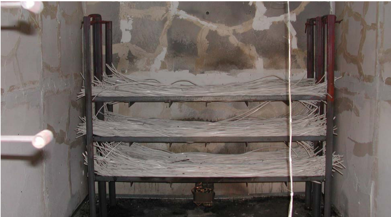
Figure 11. Photograph of Cable Trays in the Burn Room
