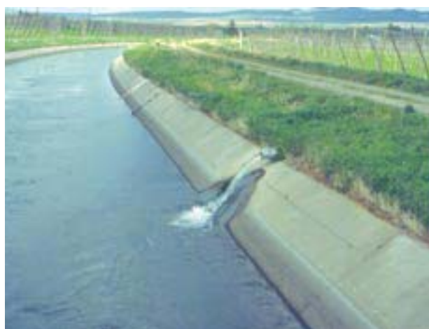
Water leaking from the Roza Canal is captured and returned by an electrical pump.
