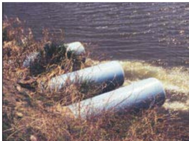
Water from a series of detention ponds is discharged to Sunnyside Canal for reuse; prior to 1998, this water would have flowed untreated to Granger Drain.
