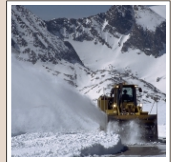
Road crews work at 12,000 feet in elevation to plow snow from Trail Ridge Road in Rocky Mountain National Park.
