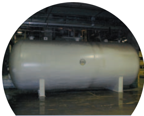
New 10,000-gallon compressed air storage tank
