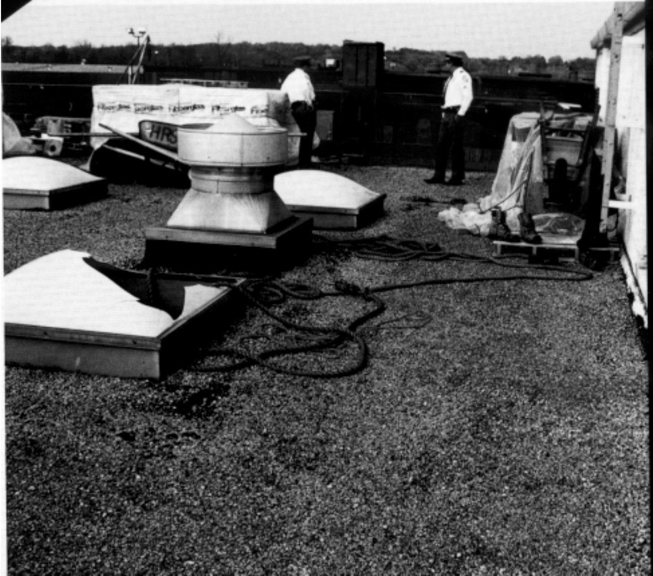
Figure 2. This Figure Shows an Intact Smoke Dome Type Skylight Just Opposite the Broken Skylight. The Fixed Ladder Providing Access to Roof of the Higher Section of the Building is Shown at Left.
