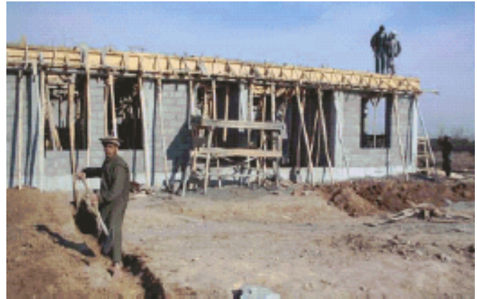
This model clinic under construction in Qala-e-Qazi is due for completion by the end of January 2004.
