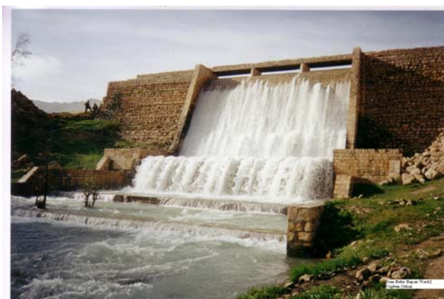
Sar-e-Haus Dam before emergency rehabilitation.
