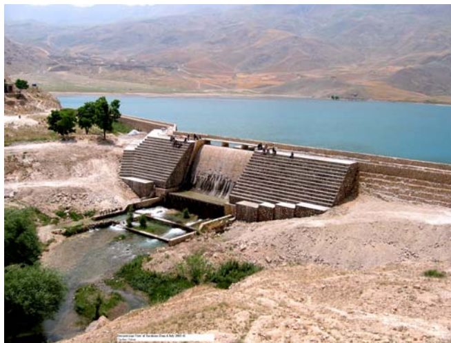
Sar-e-Haus Dam after emergency rehabilitation. Note reinforced walls added by USAID to prevent dam failure.
