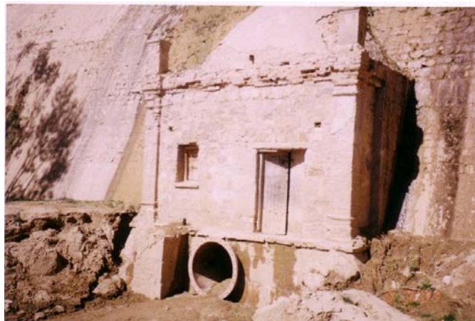
Zana Khan Dam gallery building will be repaired as part of a soon-to-be awarded contract.
