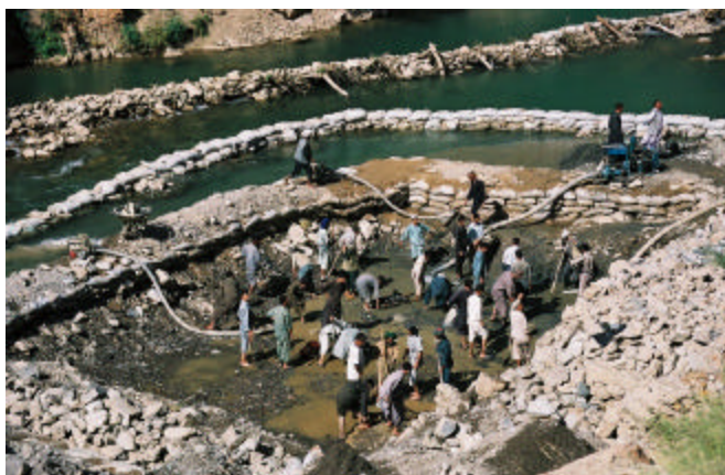
Rebuilding a diversion dam for irrigation system. Work must be done while the river's water level is relatively low in order to permit construction.
