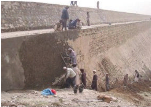
Workers begin work on the rehabilitation of Zana Khan Dam in Ghazni province.
