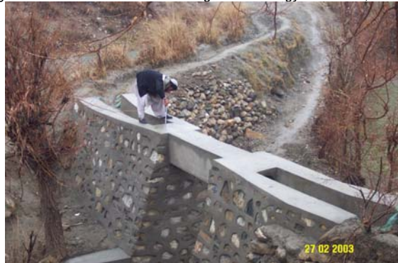
This aqueduct project allows a small irrigation canal to cross a stream in Pachir Wa Agam district, Nangarhar. Note the fine stonework done by local masons.
