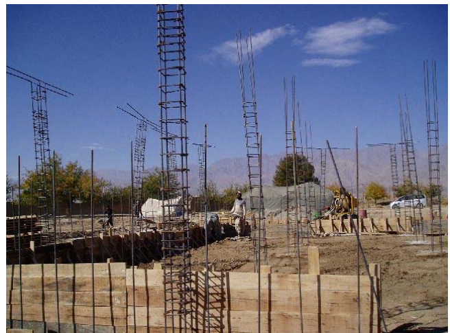
Formwork and reinforcing bar are erected for construction of this Basic Health Clinic. This past week more than 3000 bags of cement, 50 metric tons of reinforcing bar and other materials were delivered to school and clinic construction sites.
