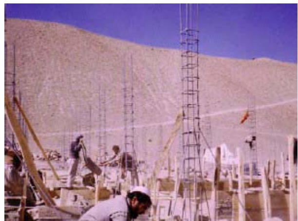
Construction on the Yakhshi School in the Nawar district of Ghazni province.
