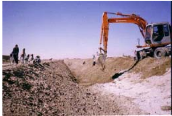
Desilting the right canal of the Sardeh Irrigation System. The right canal is 21.5 km long and irrigates 6,800 ha. It will have the capacity to convey 7.2 cubic meters per second after it is restored to its original dimensions.
