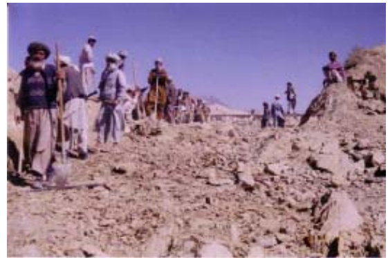
Rock excavation for the new spillway for Zana Khan Dam. The new spillway will be able to convey up to 25 cubic meters per second of water. It will be 7 meters wide and over 100 meters long when completed. It will be constructed using reinforced concrete and stone masonry.
