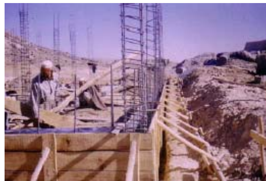
Foundation work for Tamdai Basic Clinic in Ghazni's Qarabagh district is nearly half complete
