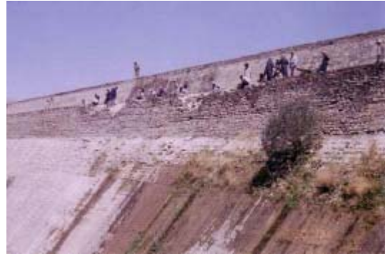
Workers repair the stone masonry on the downstream face of the Zana Khan dam.
