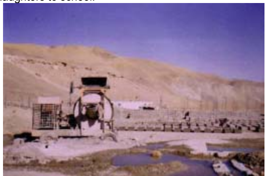
Ghulam Sakhi High School in Ghazni's Nawar district, showing 50% of the foundation completed.
