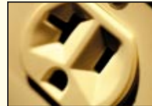
Outlets must be grounded properly.
