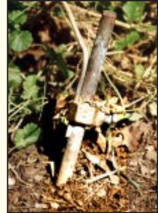
Grounding rod in the earth.
