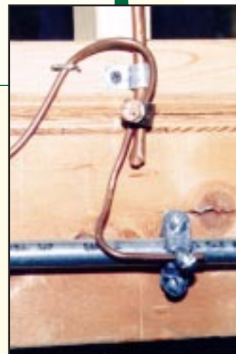
Install bonding jumpers around nonconductive material.
