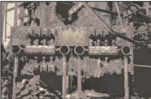
Damaged equipment can overheat and cause a fire.
