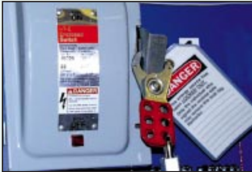
Always lock out and tag out circuits.
