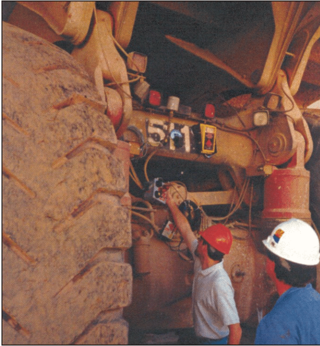
Figure 43.—Radar unit mounting position on Caterpillar 793B.
