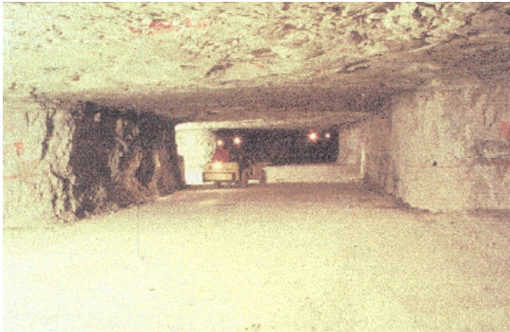
Underground view of the multiple-entry section of the Lake Lynn Experimental Mine.
