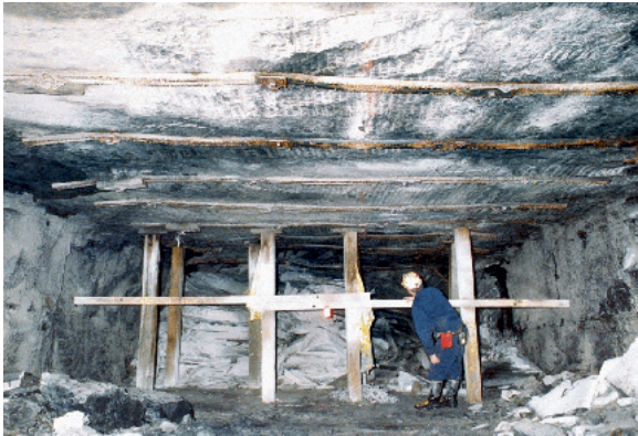
Site of fatality caused by massive sandstone roof failure in a mine in Mingo County, WV.
