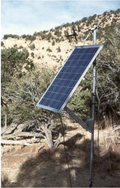
Solar panel generates energy for monitoring seismic activity in the mountains.
