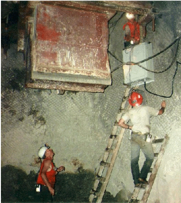
Loosening blockages in ore passes can be extremely hazardous.
