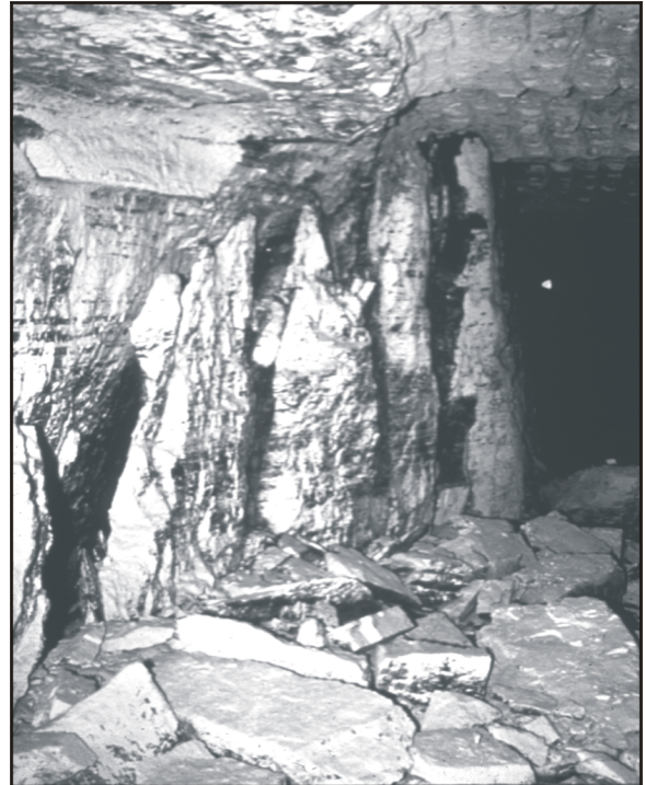
Figure 3.—Skin failure of unsupported rib.
