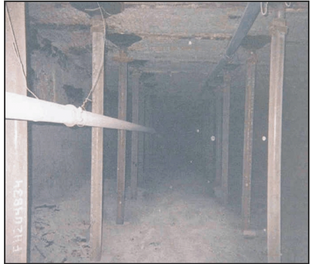
Figure 13a.—Outby area supported by ACS supports.
