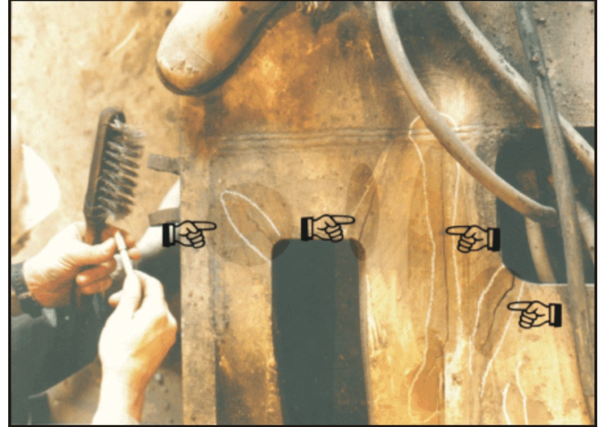
Figure 16.—Failure due to stress concentrations in cutout sections of caving shield.
