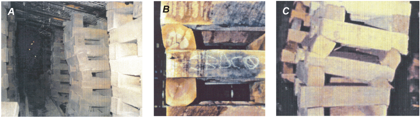
Figure 25.—Examples of poor crib construction. A , rollout of crib blocks due to inadequate overhang; B , rounded timbers degrade support; C , a single weak crib block causes premature failure of a "mixed hardwood" crib.
