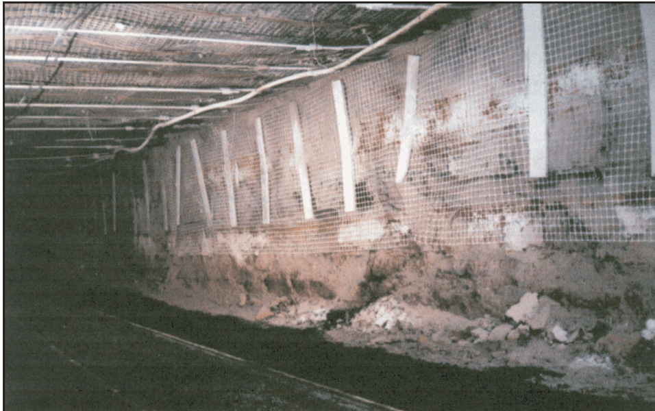
Figure 11.—Synthetic mesh supporting roof and rib. (Photo courtesy of Tensar Earth Technologies.)
