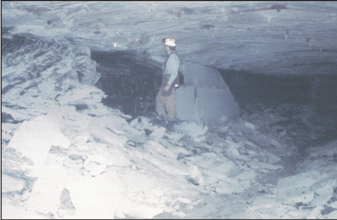
Figure 15.—Tailgate shield zone supported by cable bolts.
