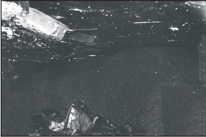
Figure 1.—Skin failure of unsupported roof.
