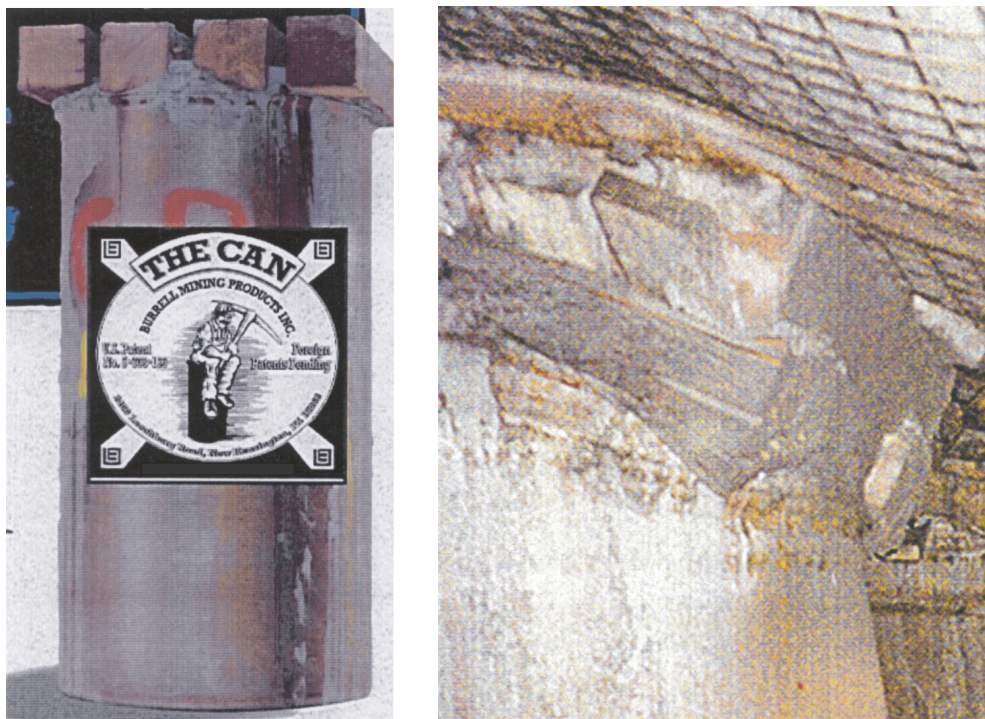
Figure 26.—Poor-quality timber on top of Can degrades support.
