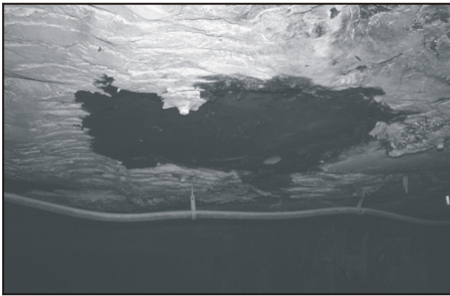
Figure 2.—Skin failure in supported roof.
