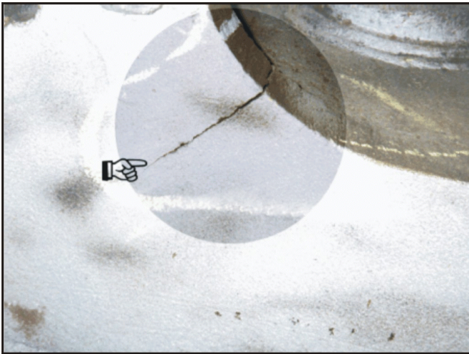
Figure 14.—Failure of base rib side plate where fabrication process left large flaws.
