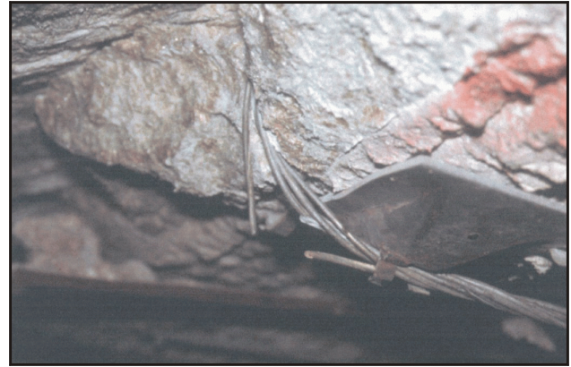
Figure 28.—Shear failure of cable truss near bearing plate.
