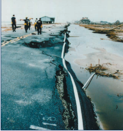
Atlantic coast hurricane causes significant damage to Barrier Island coastal highway.
