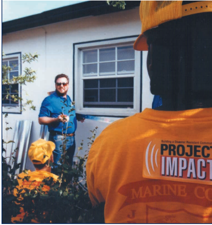
Volunteers gave up some of their time during 1998 "Spring Break" to install hurricane shutters in Deerfield Beach, Florida, a Project Impact pilot community.
