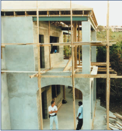
The Buccaneer Hotel in St. Croix, U.S. Virgin Islands, is constructing new condominiums to exceed current building codes for hurricane standards.
