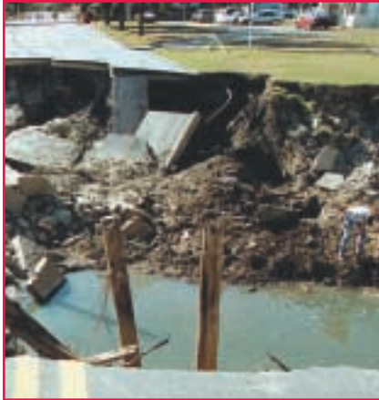
This bridge is washed out from floods, leaving this main artery unusable.
