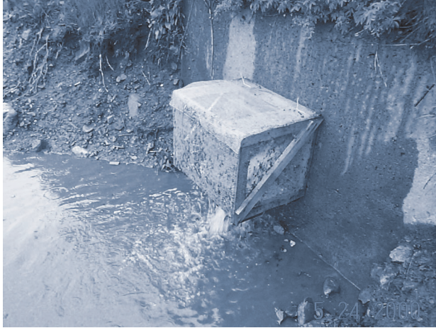
Figure 7. Debris-collection structure at the outlet of an oil-grit separator during a rainstorm on May 25, 2000, station 739, Southeast Expressway, Boston, Massachusetts.
