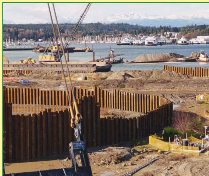
An underground sheet pile wall was installed to stop remaining contaminants from seeping into the harbor.
