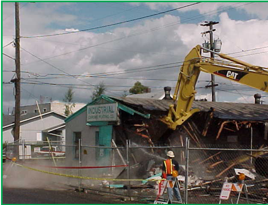
Crews demolish a Portland plating facility and remove 4,700 tons of contaminated soil and debris.
