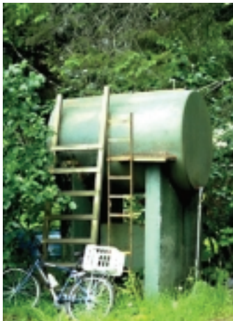
EPA's regulations covering aboveground oil storage tanks (ASTs), such as the one pictured here, are based on the concept of preventing spills through proper design, operation, and maintenance procedures.
