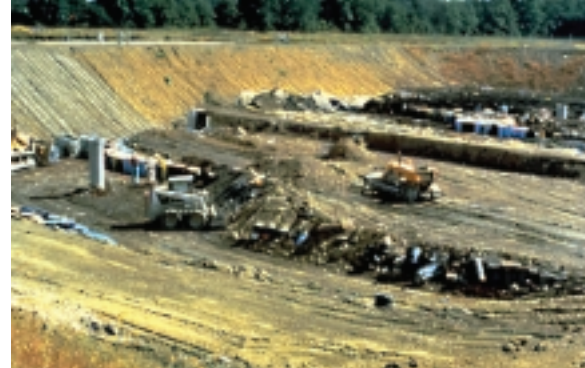
Here, personnel use heavy equipment to remove contaminated soils from a site.
