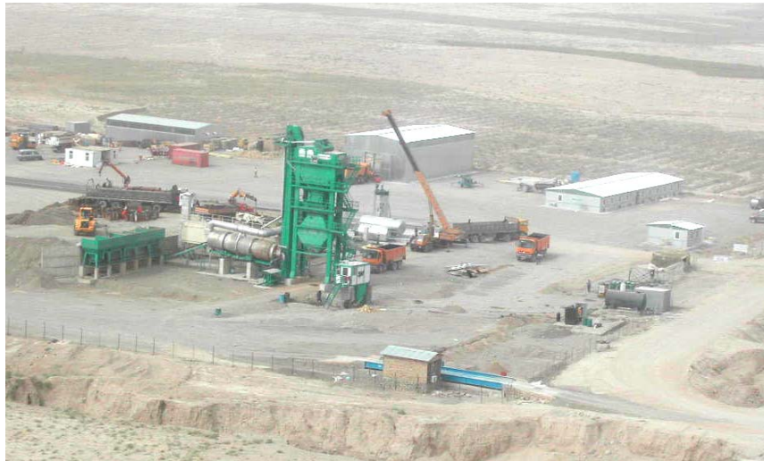
A photograph showing one of nine asphalt mixing plants being used on the Road Project. This photograph was taken in August 2003 about 390 kilometers west of Kabul, Afghanistan.
