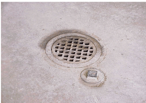
Unprotected Floor Drain Leading to Leachfield
