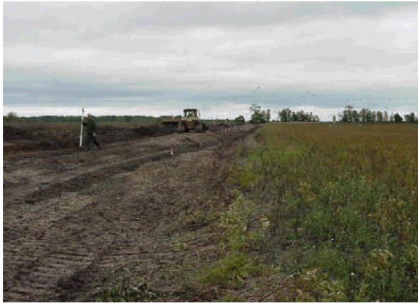
Enhancement of existing dike along the edge of the restoration project area to protect a adjacent property from flooding once part of the shoreline dike is removed. (photo by Lisa Williams, USFWS)
