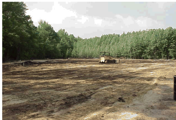
Prime Hook NWR - Post Lead Shot and Lead Contaminated Soil Removal and Stabilization - Fill and Topsoil Placement
