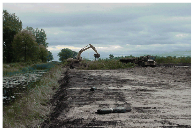
Removal of dike along access channel to Saginaw Bay. (photo by Lisa Williams, USFWS)
