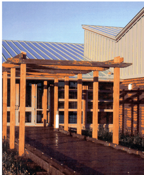
This standing seam metal roof at the Refuge is Energy Star compliant. The roof has an emissions level which meets LEED criteria for cool roofs.
