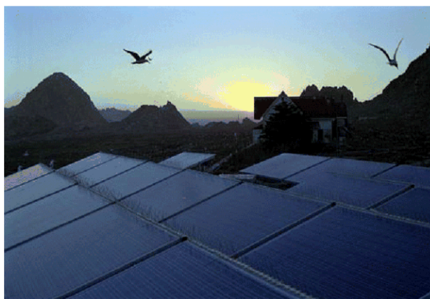
Farallon NWR Solar System
