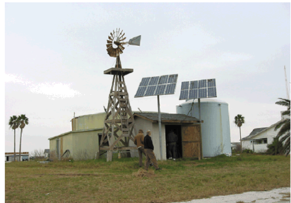
Solar Panels for Well Pumps - Aransas/Matagorda NWR
