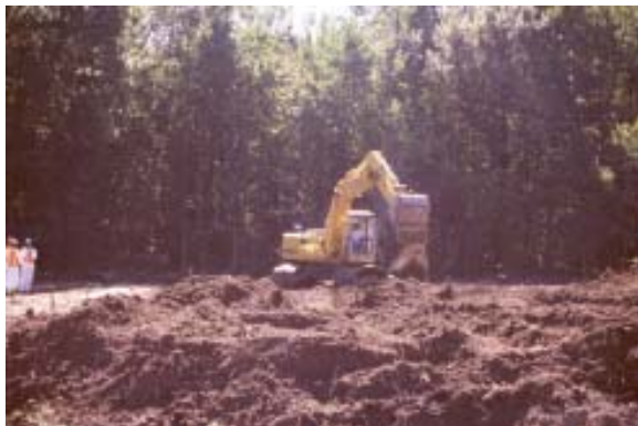
Prime Hook NWR - Excavation and Removal of Lead Shot Pellets and Contaminated Soils
