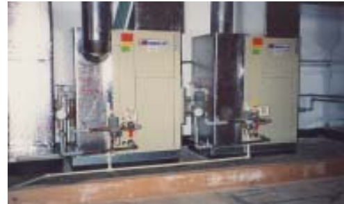
Geothermal Heat Pump Units at Creston NFH
