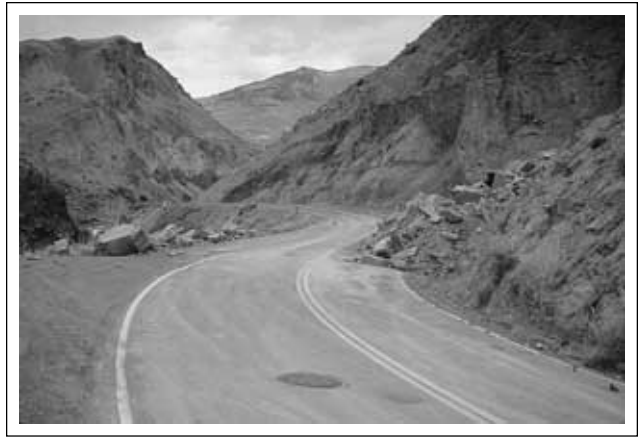
Although cultural resources were not affected by this landslide on the road between Mammoth Hot Springs and the North Entrance, the slide may bump up the maintenance schedule for this section of road. NPS photo.
