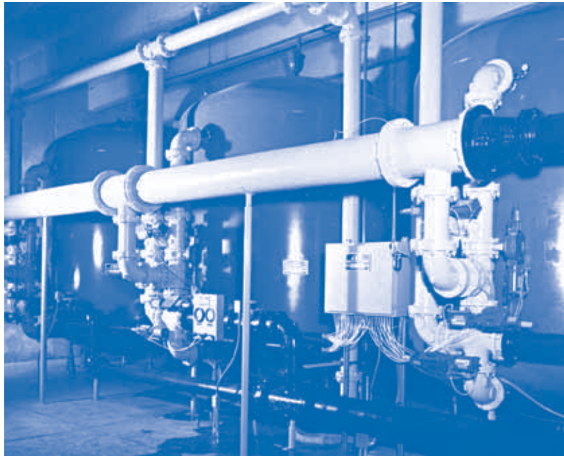
Figure 6-6. Ion Exchange System (Tonka Equipment Company).
