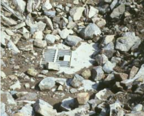
Pre-cast concrete panel closure with locking access door in the Dakota Hill project, funded in part with severance tax money from legislative appropriation
