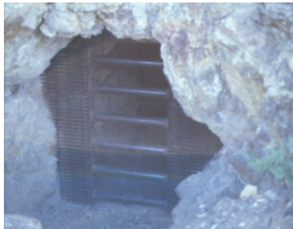
Steel grate closure with bat ladder in the Turret project, built in cooperation with the USDA Forest Service
