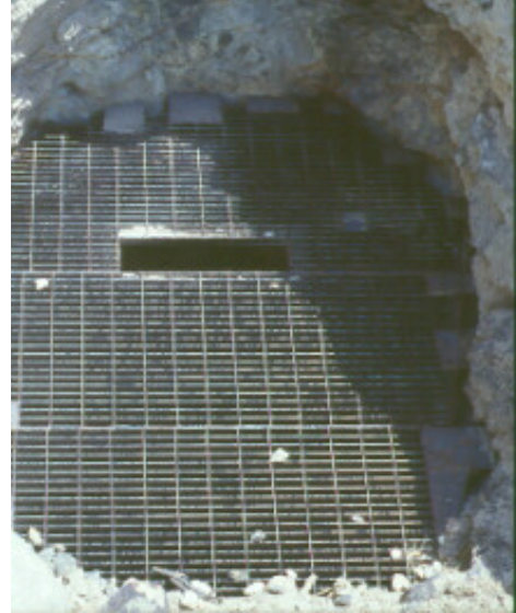
Steel grate closure with bat slot in the Turret project, built in partnership with the USDA Forest Service
