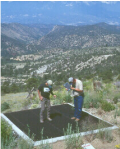
Steel grate closure with concrete footer in the Turret project, built in cooperation with the USDA Forest Service
