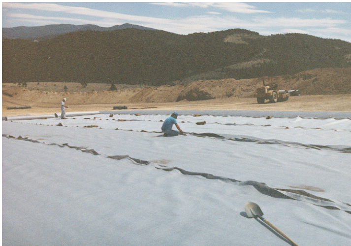
Placing the impervious liner in the repository for the Alta Mine toxic spoil.
