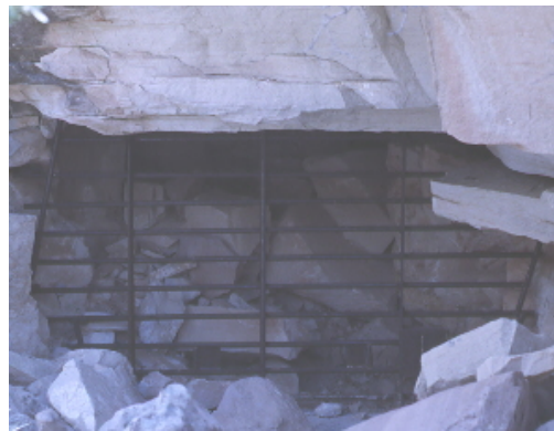
Bat gate closure in portal BH159 of the Silver Reef project – 5/11/04
