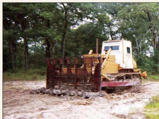
An armored bulldozer operated by U.S. Department of State contractor RONCO Consulting Corporation clears landmines along the Sena rail line. (Photo courtesy of Office of Weapons Removal and Abatement)
