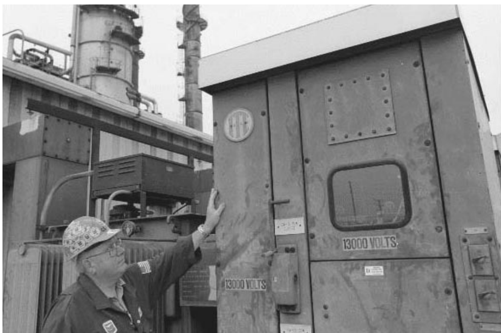
A specialist at Chevron shows where stainless steel covers have been placed atop transformer stations to stop electrical fires or shorts from occurring during heavy rains
