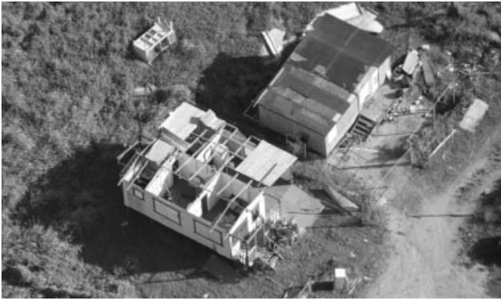
More than 65,000 homes in Puerto Rico had emergency tarps installed to replace roofs blown off by Hurricane Georges.
