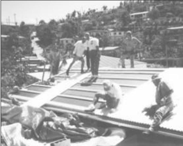
Workers in the Virgin Islands repair damage from Hurricane Marilyn which struck September 15-16, 1995.
