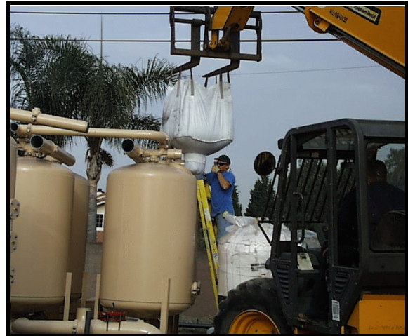
Figure 2: Loading Arsenic Treatment Media
