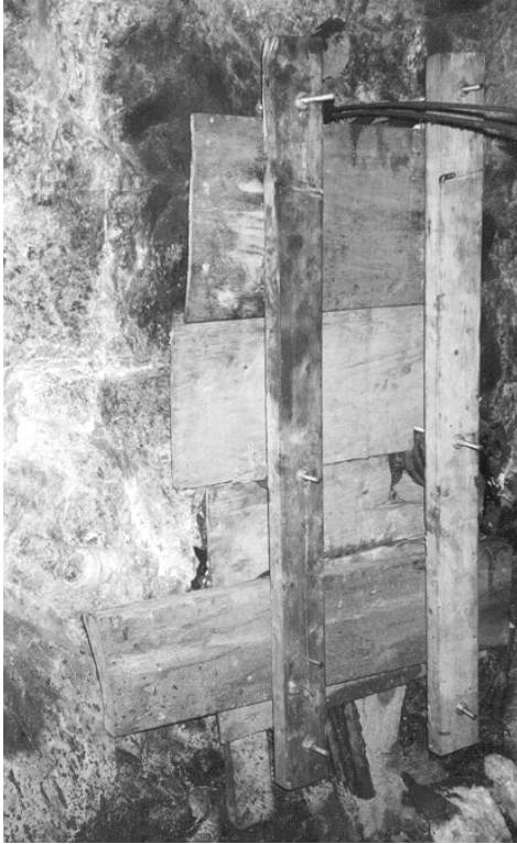
Figure A1.—Installed pressure cell.
