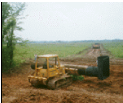
Water control structures and low dikes were installed to restore shallow water areas.
