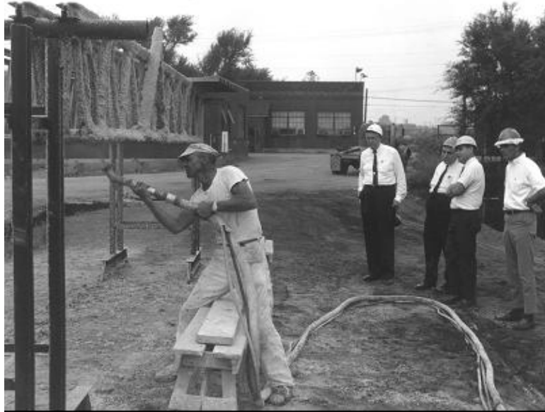
Figure 3 Demonstration of Monokote spray-on fireproofing circa 1967 at Laclede Steel Co. (Madison, Il.)
