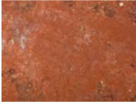
No burn faint cracks from drying of paint 1 mm
