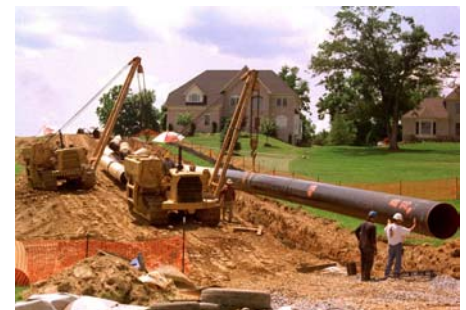
Contractors replace high-pressure pipeline in right-of-way recently encroached upon by new community.
