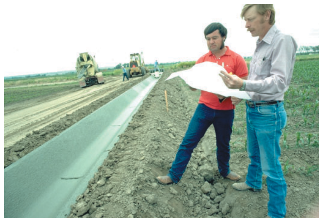
Photo 6-3. USDA technicians inspect a new concrete lined irrigation water canal that will reduce seepage and stabilize delivery. (Tim McCabe photo)
