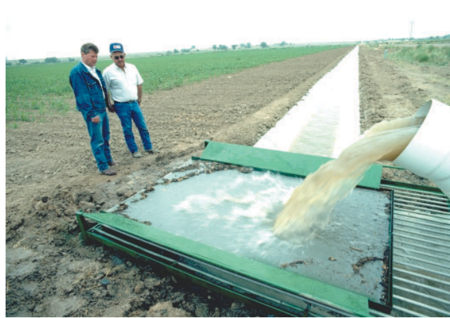
Photo 6-2. A newly installed weed rack helps keep floating debris from impeding water delivery to laterals and secondary canals. (Tim McCabe photo)
