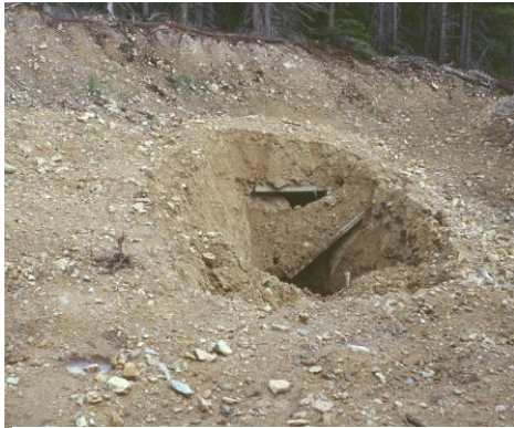
Damage to concrete panel closure in stope DH-14 of the Dakota Hill project, requiring maintenance
