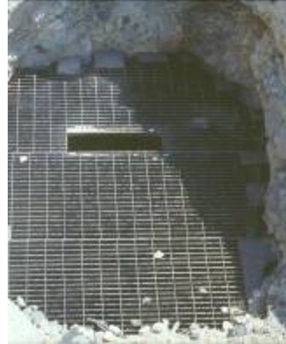
Steel grate closure with bat slot in vertical opening #112 of the Turret project
