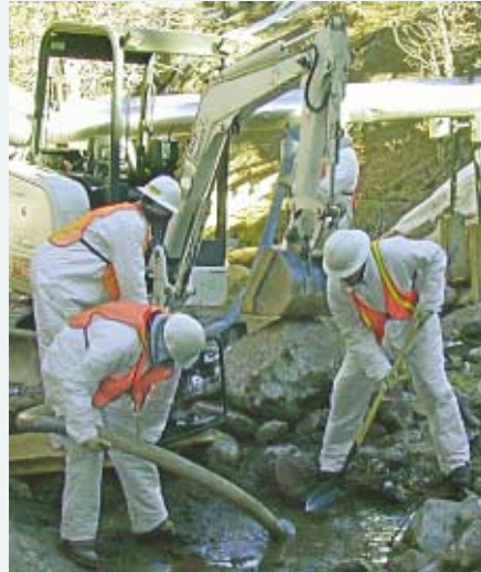
Left Some contaminated soil and water must be removed by hand, using shovels and vacuum equipment. Workers wear protective clothing and are monitored frequently for radiation and other potential contaminants.
