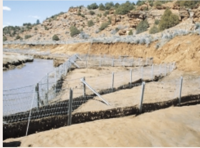
Figure 4.17: Recently installed treatment. (April 1987.) Porous fence revetment designed to reduce bank failure.
