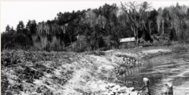
Figure 6.12: Brushmattress and plantings after spring runoff in March 1938. Note pole jetties. Brushmattressing involves applying a layer of brush fastened down with live stakes and wire.
