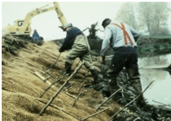
Figure 6.7: Installation of erosion control fabric. Installing measures can be considered a “mid-point” in restoration and not the completion. Preceding installation is the necessary planning, with monitoring and adaptive management subsequent to the installation.
