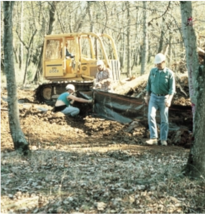
Figure 6.14: Workers installing a silt fence. Familiarity with on-site conditions is critical to successful implementation of restoration measures.
