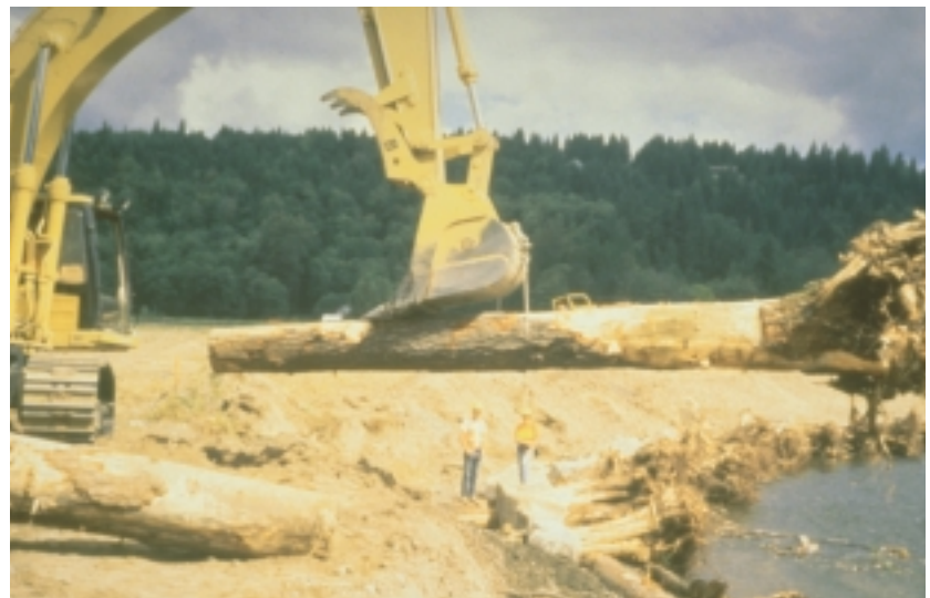
Figure 8.43: Installation of logs with intact root wads. An advantage to using tree revetments is the creation of habitat for invertebrates and fish along the streambank.
