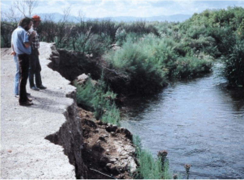
Figure 8.38: Eroded bank. Preliminary site investigation and analyses are critical to successful streambank stabilization design.
