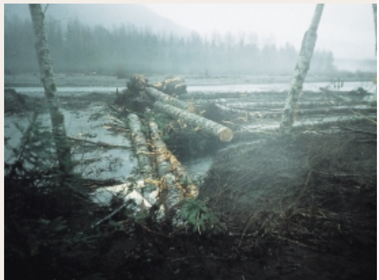
Figure 9.23: Engineered log jams. Engineered log jams (ELJs) can restore riverine habitat and in some situations provide effective bank protection.
