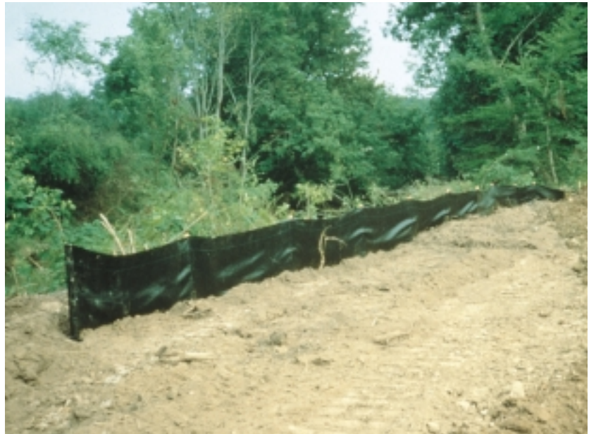
Figure 9.2: Silt fence at a construction site. Properly chosen and installed silt fences can provide a significant degree of off-site sediment control.
