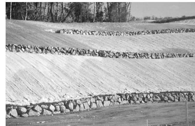
Terracing can be used to slow runoff. Lined diversion ditches direct flow away from exposed areas toward stable portions of the site.
