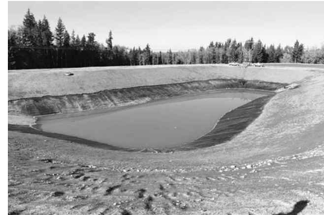
Lined sediment basins are used to collect runoff from disturbed areas on construction sites and allow heavier solids to settle out.
