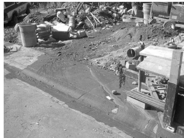
Improper management and disposal of wastes can result in polluted storm water discharges.
